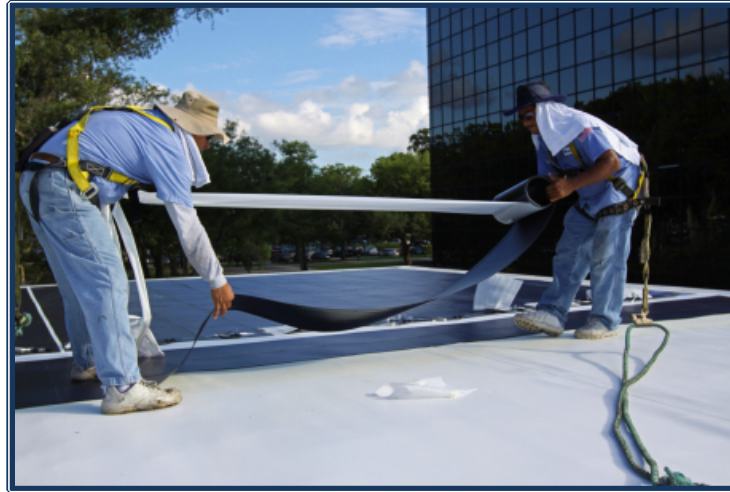
Solar Energy Management workers install flexible, thin, lightweight solar panels on the roof of Aurora's Headquarters 19329 U.S. 19 N. in Clearwater.
